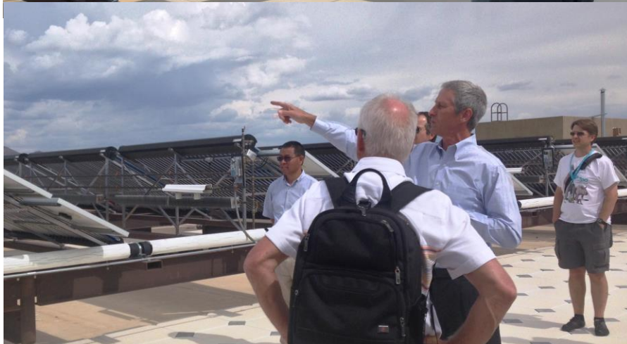
Luke Spangenburg showing the solar-thermal system to Dr. Yan, Dr. Lammers and Dr. Hanson
