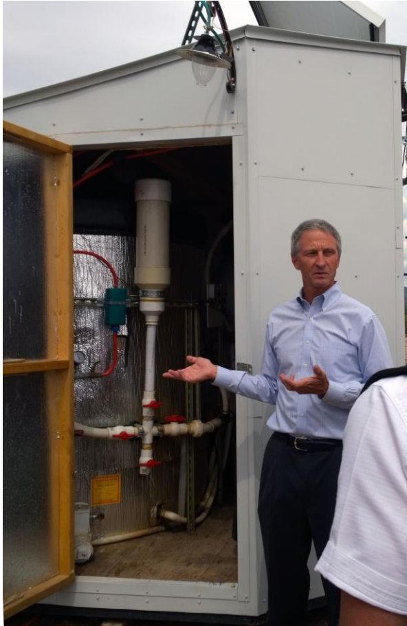
Luke Spangenburg showing the anaerobic digester at SFCC
