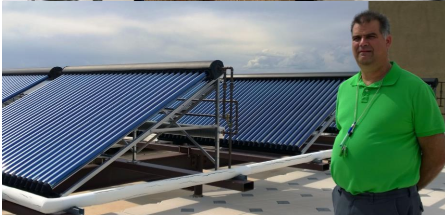
The solar-thermal collection system on the roof of the Sustainable Technology Center at SFCC. Dr. Gómez for scale
