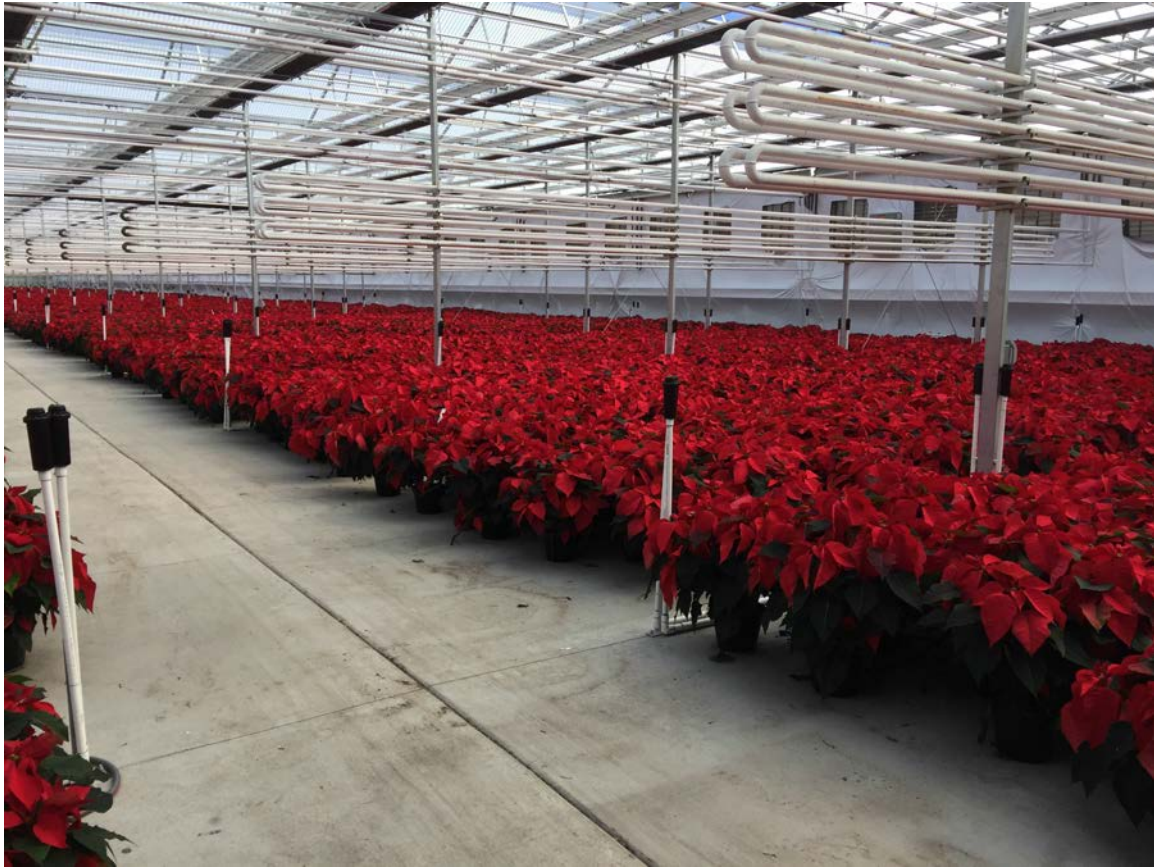
Figure 1. Inside view of Mason-Radium Springs 20-acre geothermal greenhouse. Looped pipes above plants circulated fluids heated by brackish geothermal waters. Heat exchangers transfer heat from the geothermal fluids to a freshwater loop used by the greenhouse.
